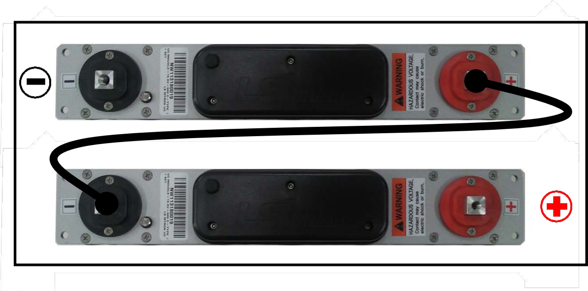
<Fig. 2> Series Connection of Modules
